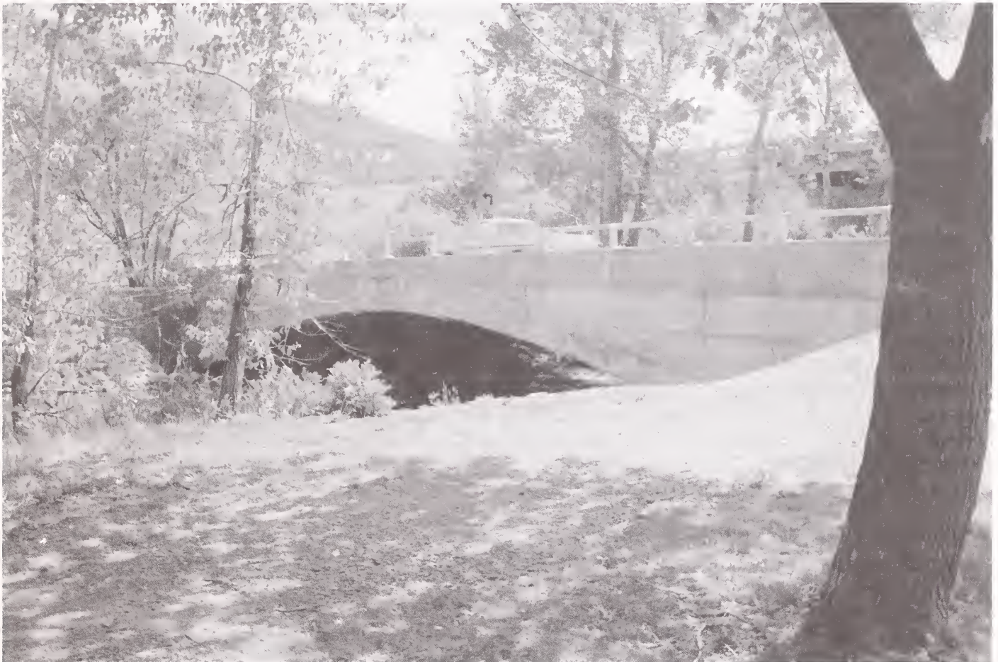
The Vine Street Bridge was the last reinforced concrete arch structure built by the Montana Highway Commission.
